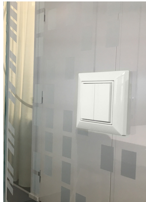
Wireless Control Panel mounted on a glass wall.
